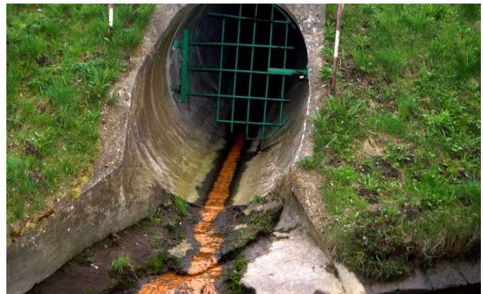
Potential illicit discharge flowing out of a concrete outfall. Confirming an illicit discharge may require sampling or other investigative methods to determine the pollutant and responsible party.
